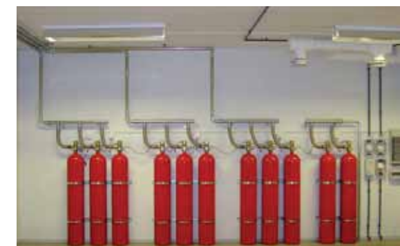
Computer room at University of Lund Sweden: Library protected with Clean Agent FS 49 C2
